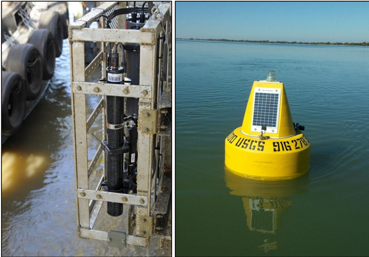
Figure 2-2. (L) shows a Sea-Bird Coastal SUNA V2 (Submersible Ultraviolet Nitrate Analyzer) mounted on a fixed structure on the Mississippi River at Baton Rouge, where the instrument cage is lowered and raised. (R) shows a NexSens buoy supporting a Sea-Bird Coastal SUNA nitrate sensor and WET Labs Cycle Phosphate sensor (in addition to a YSI EXO multi-parameter sonde measuring algal pigments, turbidity and dissolved organic matter). (Photos courtesy of Brian Pellerin/USGS)
